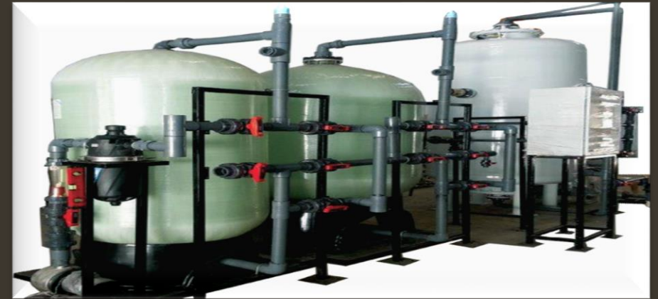
DM WATER PRODUCTION UNIT CAPACITY : 50 M 3 /HR
